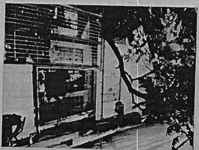
BAGONG ILOG C.D.C. SCOPE: REPAIR OF KITCHEN CABINET & MAIN DOOR, REPLACEMENT OF FACET, REPAIR OF KITCHEN SINK, REPAIR OF BATHROOM, REPAIR OF CEILING INSIDE CLASSROOM, INSTALLATION OF SIGNAGE
